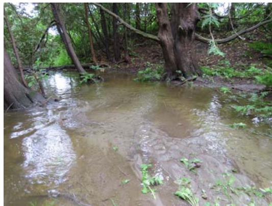
Left: Failing Wing Deflectors in Shields Creek Above: Sediment loading
