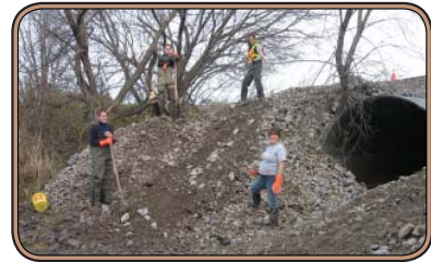
SNC staff and volunteers work hard to move rocks around the Stark Drain.
