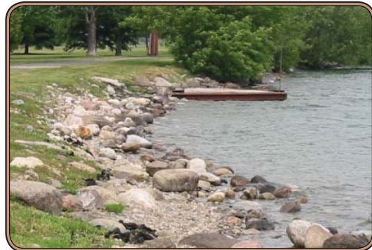
Morrisburg shoreline prior to erosion repair.
