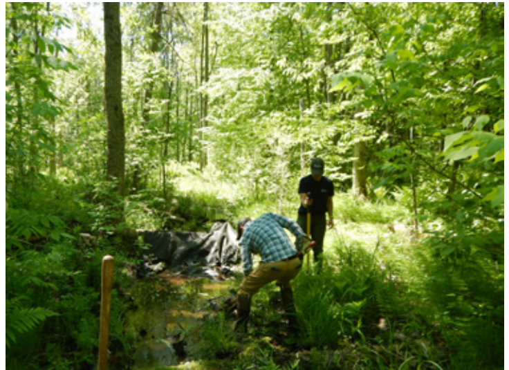
Building Beaver Dam Analogs at wetland restoration site, Township of Alfred and Plantagenet
