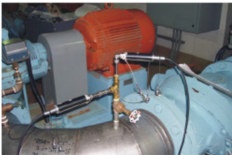
Thermodynamic testing to measure pump efficiency. Source: Hydratek.
