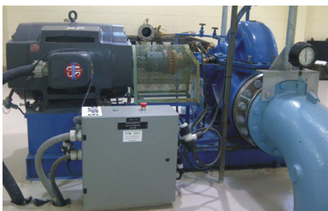
Motor and pump at a pumping station in the Region of Peel
