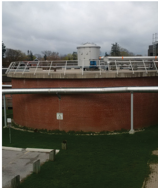
Anaerobic digester at City of Barrie Wastewater Treatment Facility. Source: City of Barrie.
