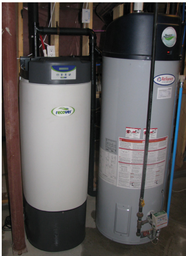
Greywater tank for domestic water reuse (on left). Source: Region of Durham.
