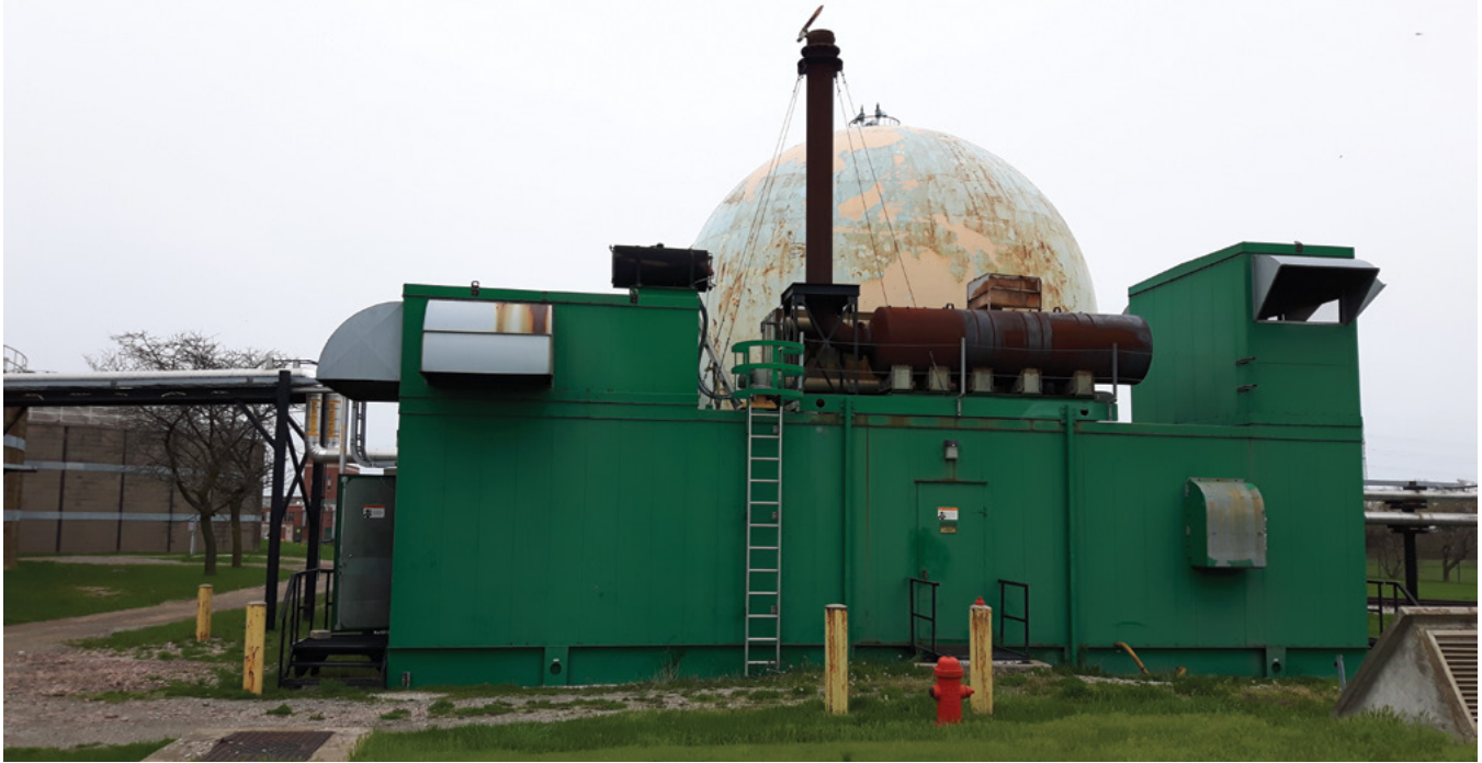
Hamilton biogas storage sphere and co-generation equipment. Source: City of Hamilton.
