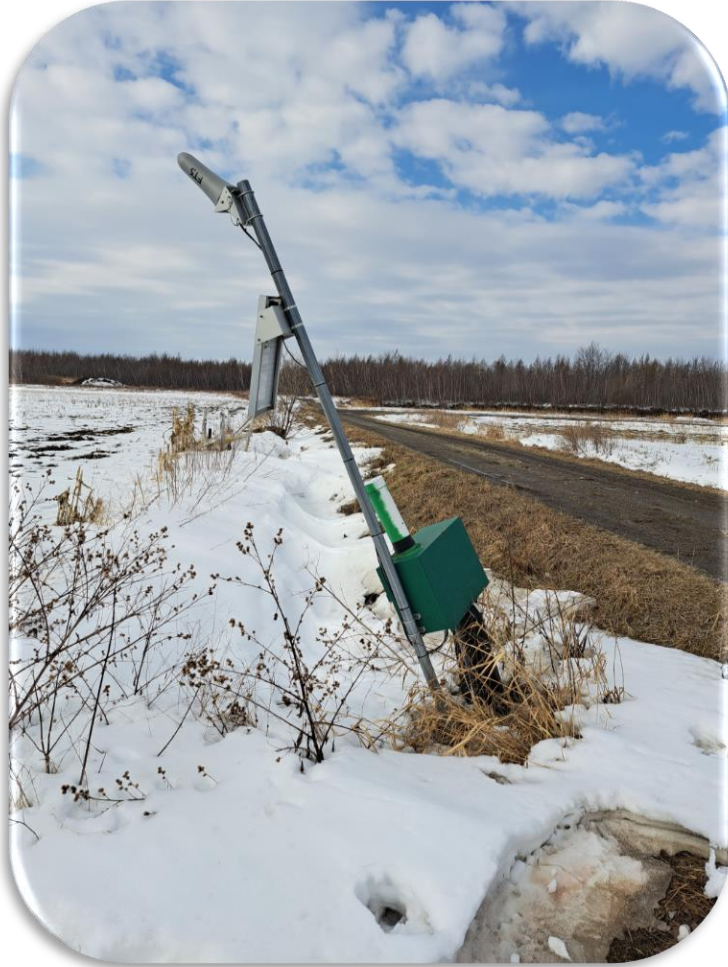
Damaged PGMN Box, Alfred Bog (April 2024)
