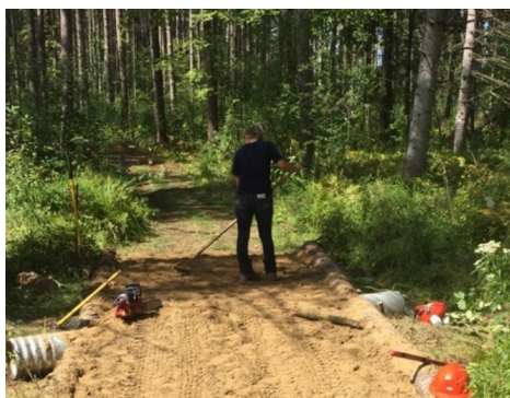
Trails at the Robert Graham Conservation Area in South Dundas were resurfaced and new culverts were installed to help alleviate seasonal flooding.
