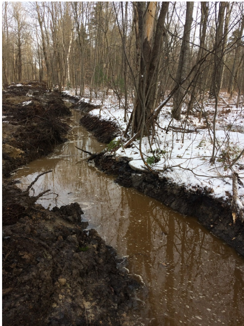
Figure 14 Excavation works created meanders in the channel to help recreate natural shaping caused when water levels are high. This will typically take place during the spring freshet.
